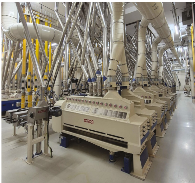
Ocrim new milling plant installed at Molini Valente.
